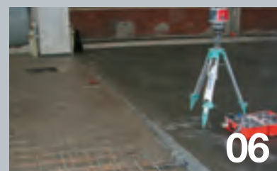
Concrete can be on both side of Ideal Joints at the same time or alternate days to separate two placements.
