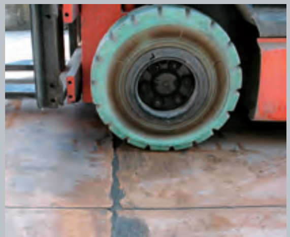
Example of construction joint damaged after a few months of life
