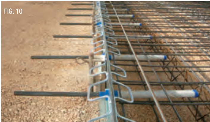
FIG. 10 Detail of Ideal Joint System® installed and ready for the concrete placement.
